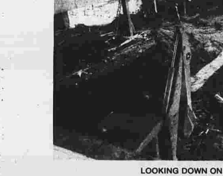
LOOKING DOWN FROM THE FIRST FLOOR ... work is still far from completion
